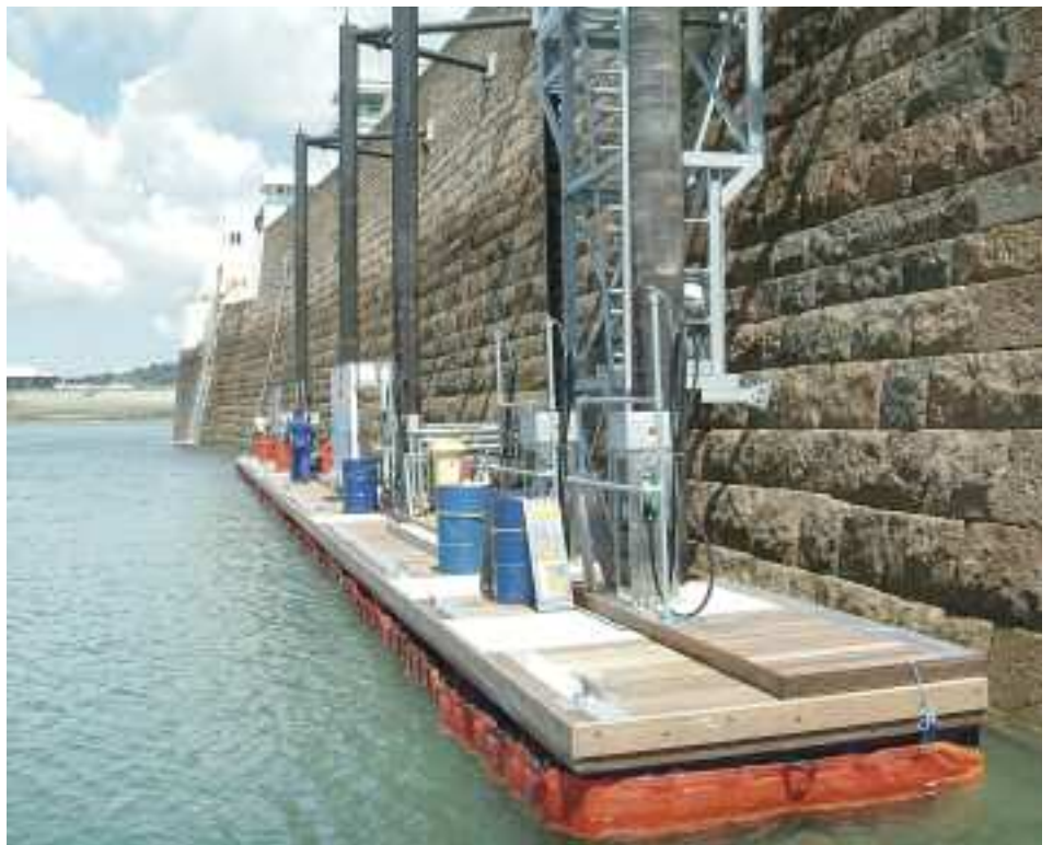
The new refuelling system at St Helier, Jersey
