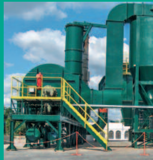
The thermal desorption plant
